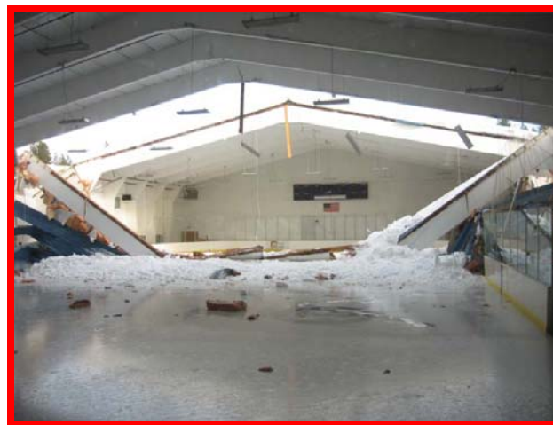
US Rink Collapse 2009
