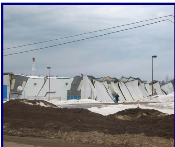
Fort Nelson Arena Collapse 2007
