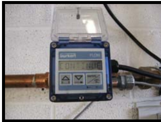
Figure 3: Computerized water valve (Town of Milton)
