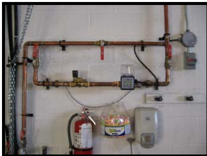
Figure 4: Computerized water valve system (Town of Milton)
