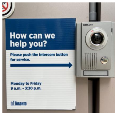
Sample intercom/camera equipment and process to eliminate entry of non-essential individuals
